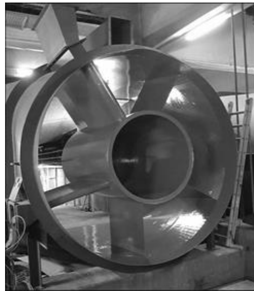
Figure 9: Fan casing after treatment
