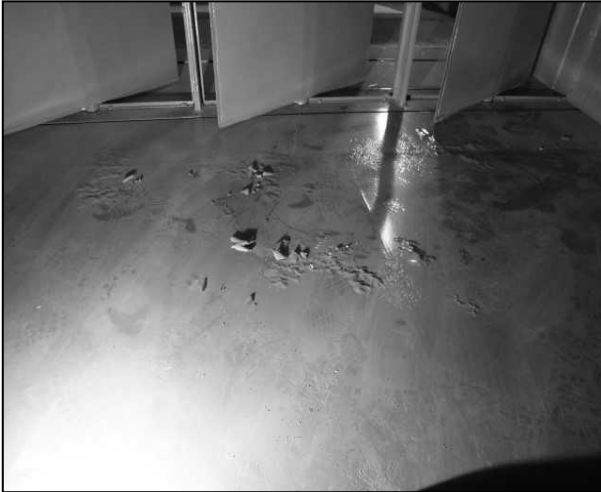
Figure 10: Delamination after treatment
