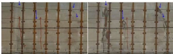
Figure 4 Evolution of water seepages (left: 2021, right: 2022)
